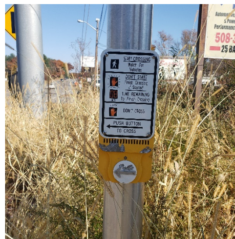
Figure 6: Controlled Pedestrian Signal
