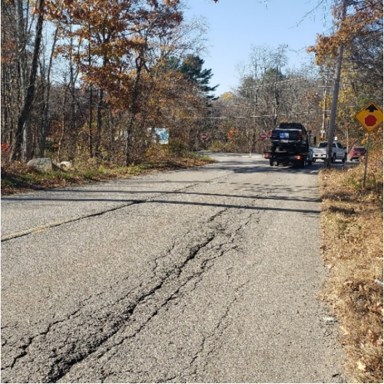
Figure 23: Pavement on Cedar Hill Road in Marlborough
