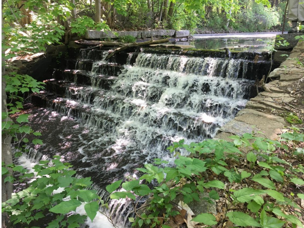
Figure GG-5 Dam for the Northborough Reservoir in Shrewsbury (Photo courtesy of Norm Corbin)
