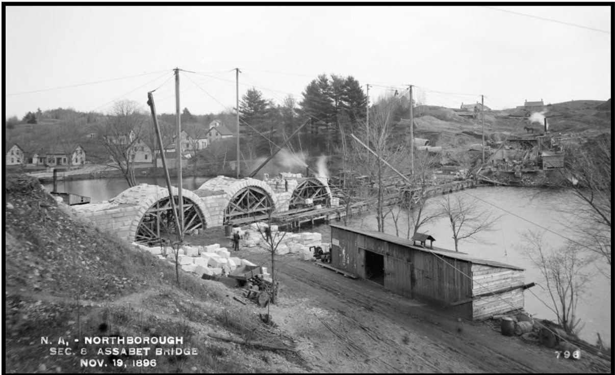
Construction of the Aqueduct over the Assabet River November 19, 1896 (Photo Courtesy, Digital Commonwealth)
